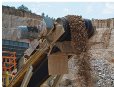
Fig.1. Motor at a conveyor.
